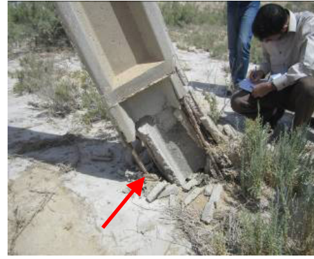
Figure 4. Concrete crushing in 20kv overhead pole
