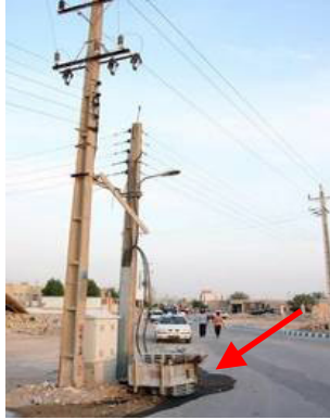
Figure 3. Falling of overhead transformer
