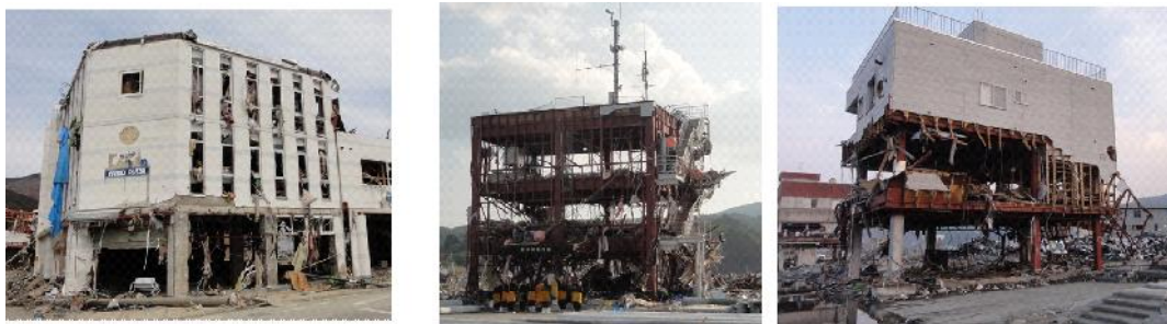
Figure 1. Typical tsunami damage to RC and steel-frame buildings observed in our field survey after the 2011 Tohoku earthquake. The damage was concentrated to exterior walls and lower stories of buildings
