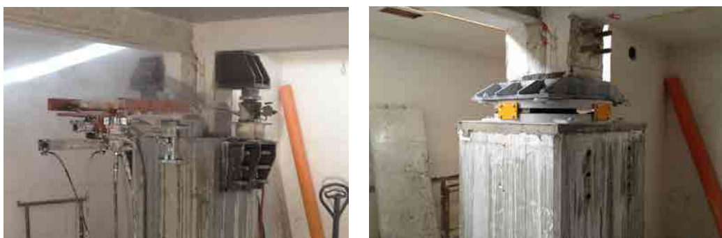
Figure 1. One of the phases of the intervention for installation of an isolator in a R.C. Column (left); a curved surface slider as installed in a R.C. Column of an existing building in L'Aquila, Italy (right)
