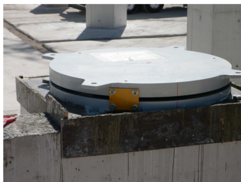
Figure 1. A double concave curved surface slider during installation in the Van Medical Campus (Turkey)
