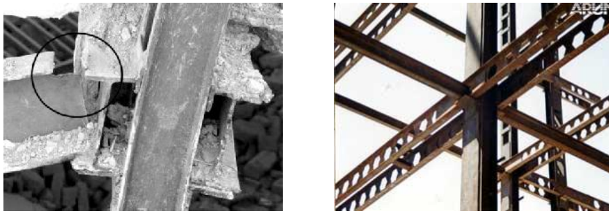
Figure 1. Reported brittle connection failure and roof collapse at Bam earthquake, 2003
