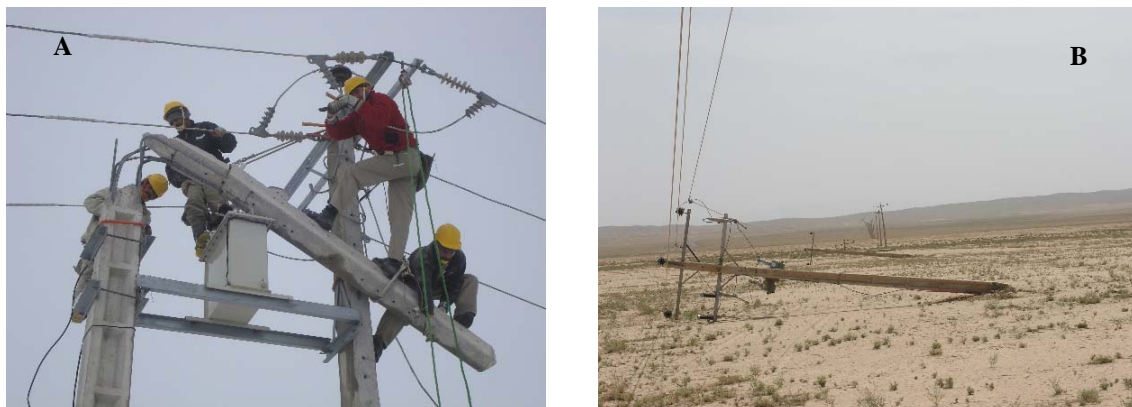
Fig.4. (A) Repair in NKEDC after a flood, (B) Failed power pole due to the flood
