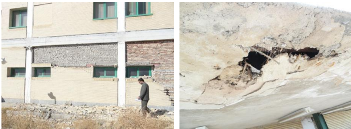
Figure 5. Failure of façade (left), and failure of metal meshes coated by plasters in a suspended ceiling (right)
