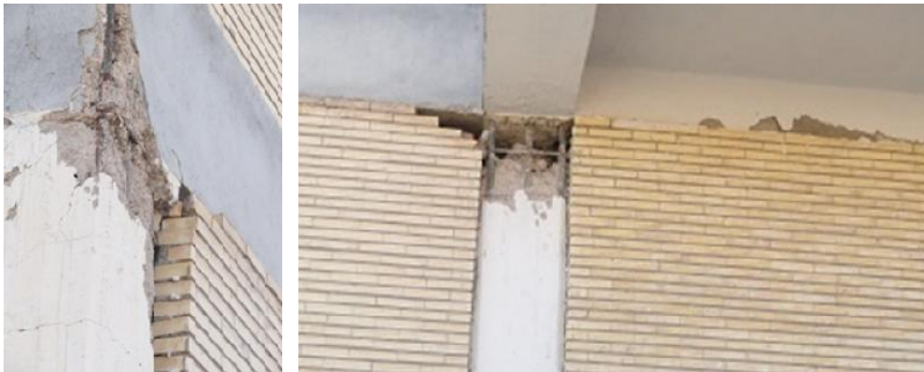
Figure 1. Shear cracks and plastic hinges in columns and cracks in beams due to the presence of infill walls
