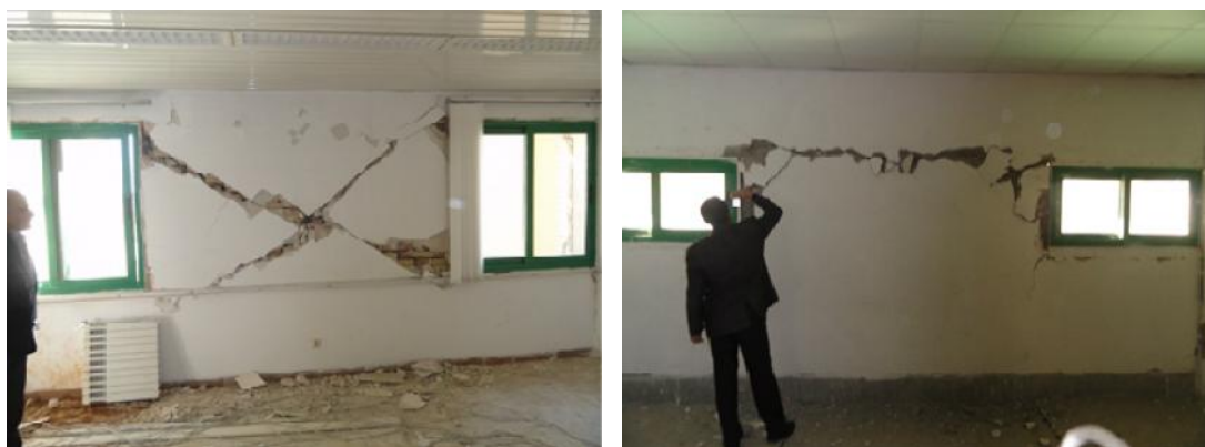
Figure 2. Typical cracks in structural infill walls
