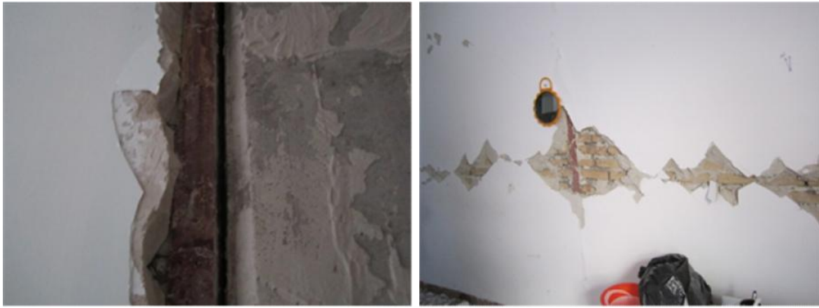
Figure 3. Double angles at the edge of non-structural infill wall (left) and spall of plaster at the middle of infill wall showing the mid-span angles used there (right) (Consulting Engineers of Fadak, 2013)
