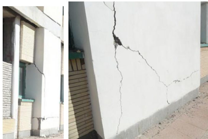
Figure 4. Typical cracks in non-structural external walls
